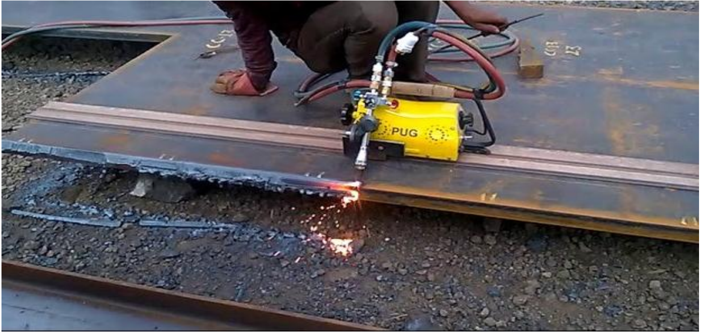
Steel Plates Cutting Area
