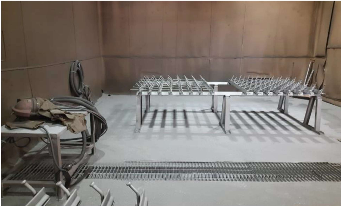
Shot Blast Room
